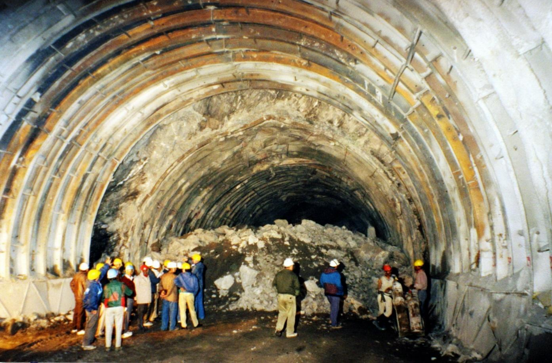
Squeezing of a headrace tunnel top heading in the Daj Khad fault zone, Nathpa Jhakri Hydroelectric Project, Himachel Pradesh, India
